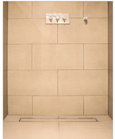
■ After completion – the shower was tiled with fine stoneware, and anti-slip material was used for the floor covering.
