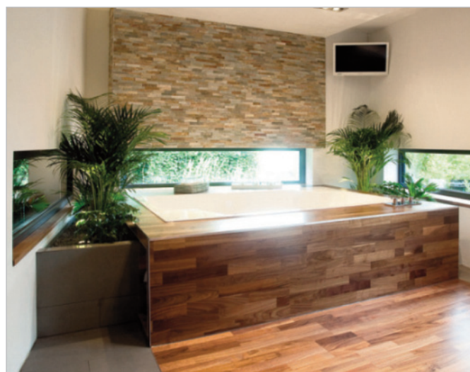
■ After completion – the bath tub area is surrounded by walls on three sides and has a very sophisticated real walnut parquet cladding.
