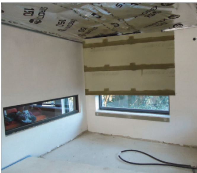
■ Implementation – the 18 m 2 large room was completely re-designed and the long, rectangular windows newly installed.
