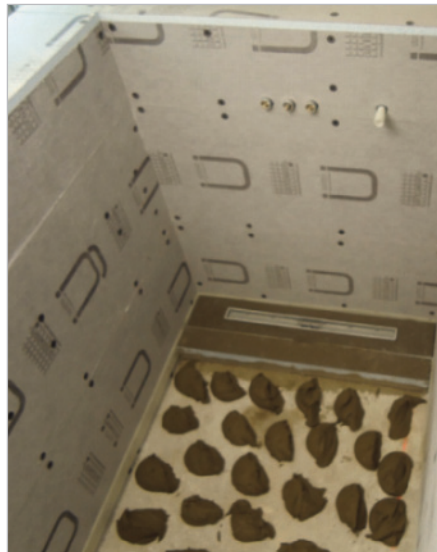
■ Gradient elements were processed in the flush with the floor shower with the drain channel using the "dot technique".
