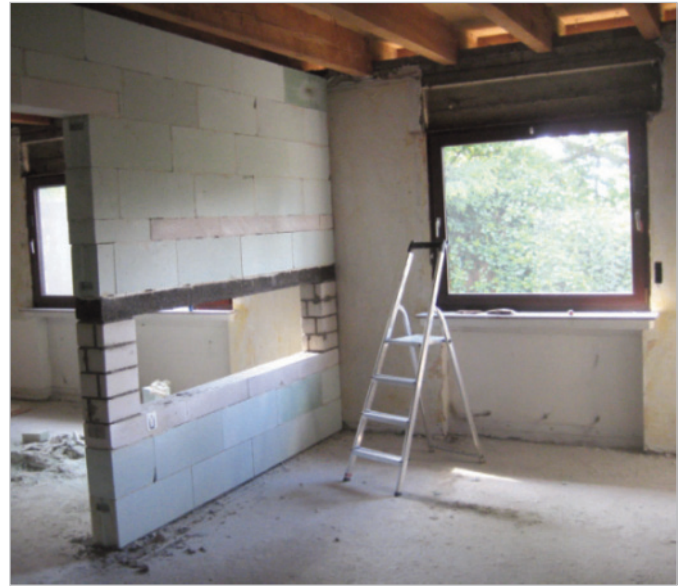
■ Before – when it all began: the Franks built their dream bathroom from scratch.
