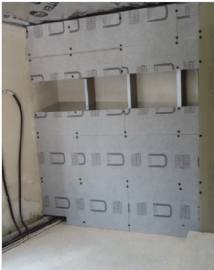
■ In the shower area, factory-sealed construction panels were applied to a substructure in rib construction.
